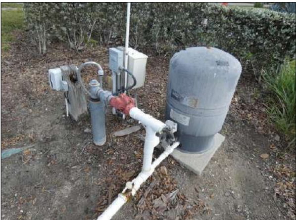
Well and Pressure Tank
