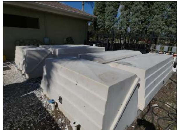
Pool Equipment Housing Boxes
