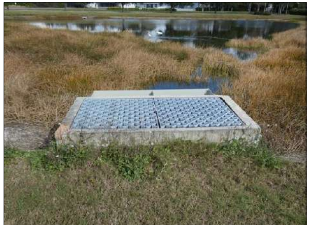
Stormwater Drainage Control Structure
