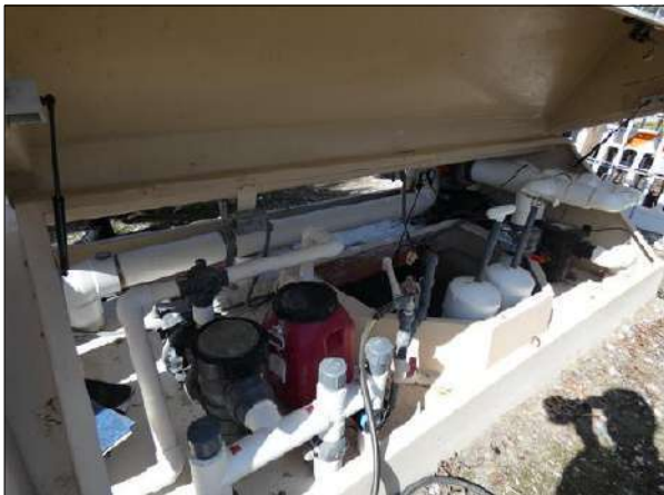
Pool Pumps and Equipment
